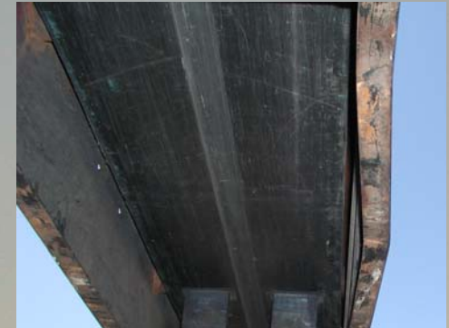
Damaged Crane Structure
